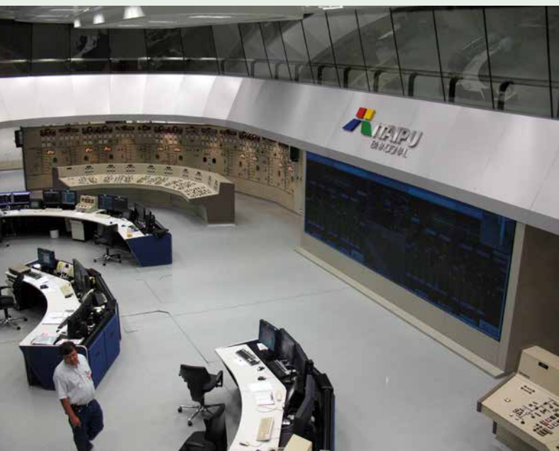
Left: Control room at Itaipu. (Photo: Anagoria / Wikimedia CC BY 3.0.) Right: Substation at the Itaipu Dam.
